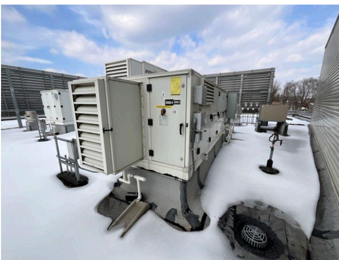
29 - TYPICAL ROOFTOP PACKAGED UNIT
